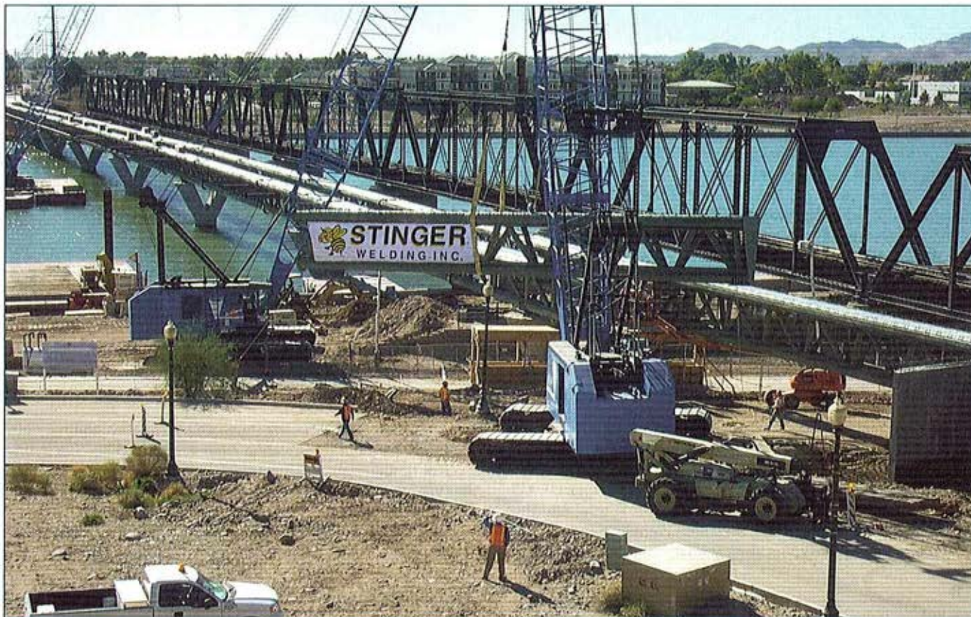
Fig. 1 — The bridge services the Phoenix, Ariz., light rail network and spans Tempe Town Lake. Here the last segment is being hoisted for setting at the northeast abutment. At right, parallel to the new bridge, is the historic 1912 single-track truss bridge that is still in use.
