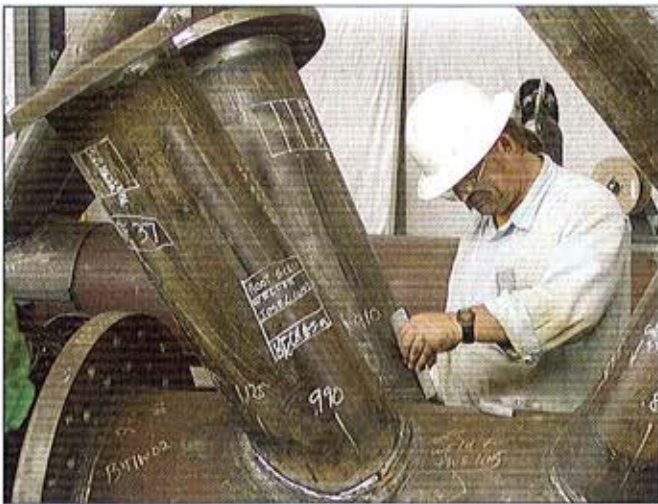
Fig. 4 — UT technician and CWI Dennis McNamara verifying depth of groove after grinding a root pass.
