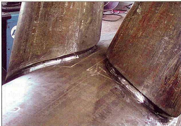
▲ Weld Done. Phoenix steel truss light-rail crossing required complex pipe cutting and welding for 722 unique pieces of diagonal bracing that demanded tight tolerances.
